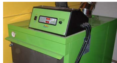
ELECTRICAL PANEL ON BOILER
